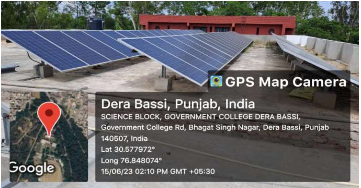
Grid connected Solar PV Plant installed in GC Dera Bassi Campus
